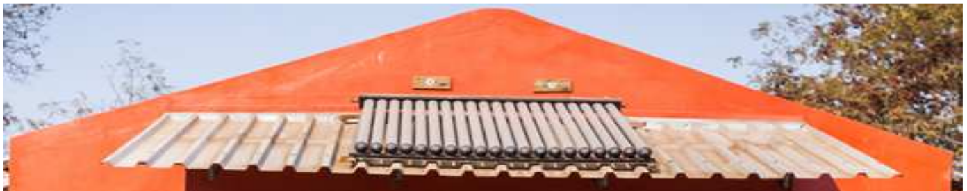
Solar hot water waiting for us to connect it for them ... and now we WILL
